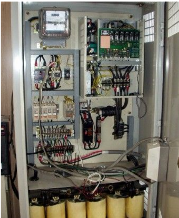
Pic.4, 3 phase inverter
