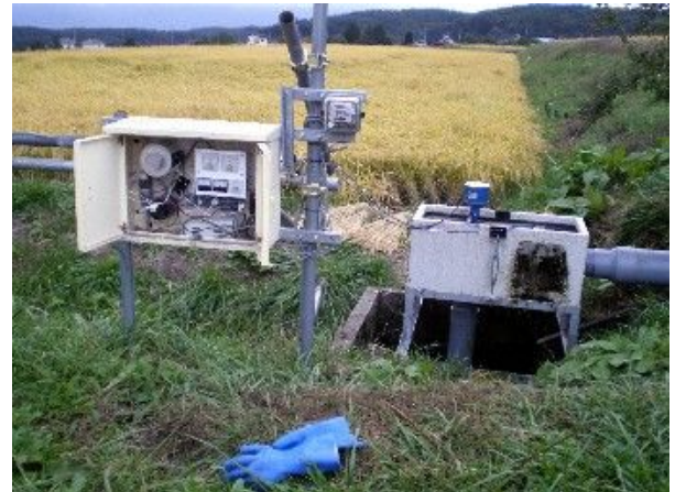
pic.5 control box
