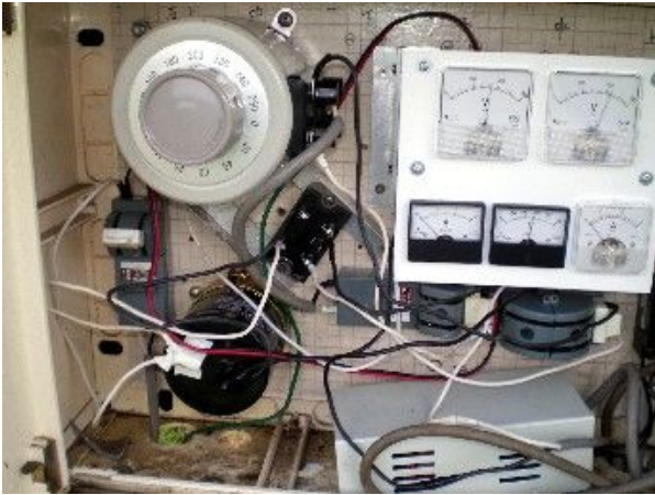
pic.6 control box
