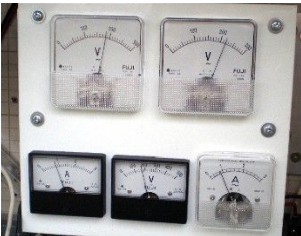
pic.7 panel meters
